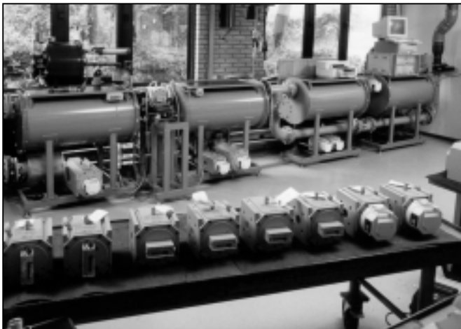
Figure 6. Rotary meter calibration facility - The Netherlands.
